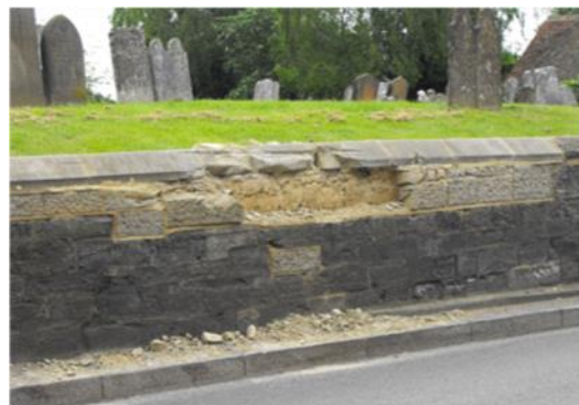
Figure 54 Damage to listed buildings
